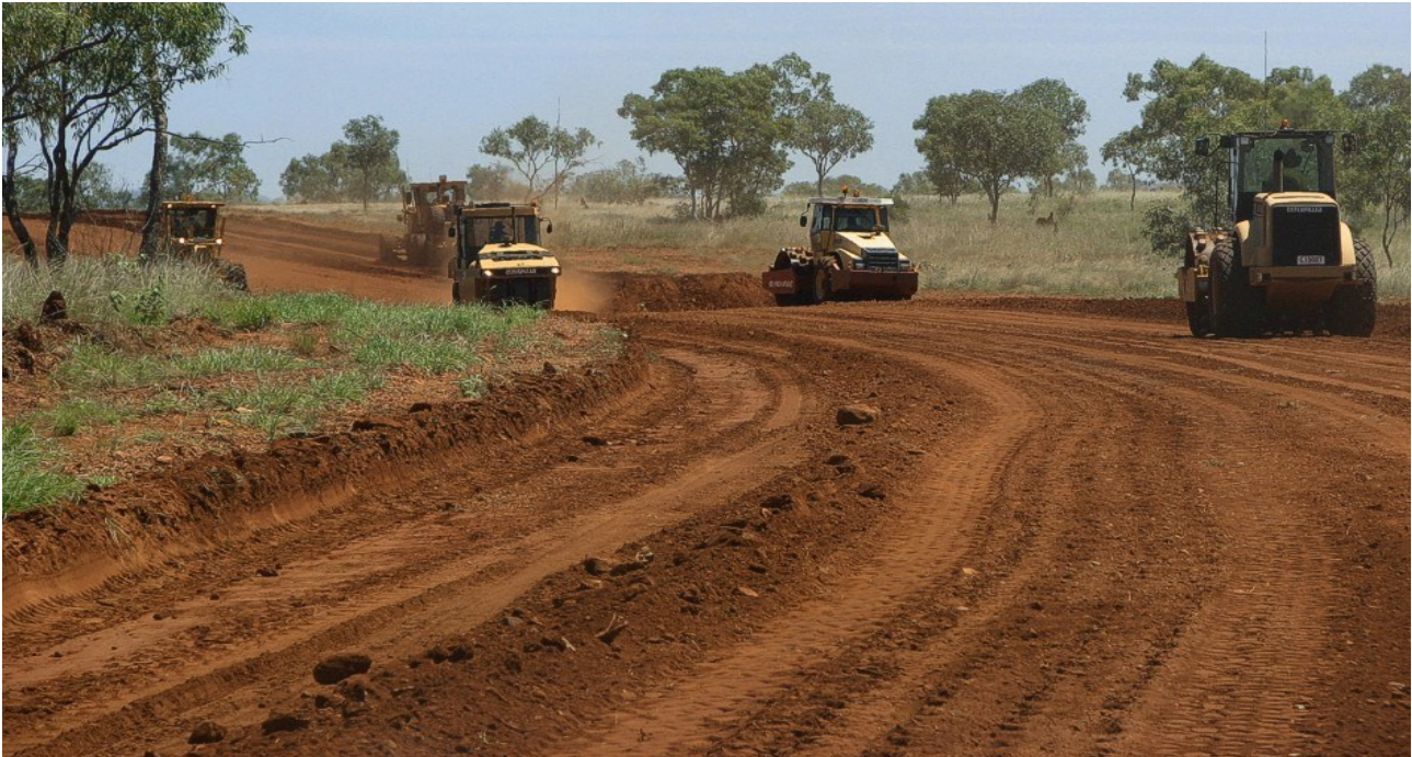
Fig 8: Major road works have commenced on the main access road connecting the Rocklands Site to the Queensland Highway grid.
